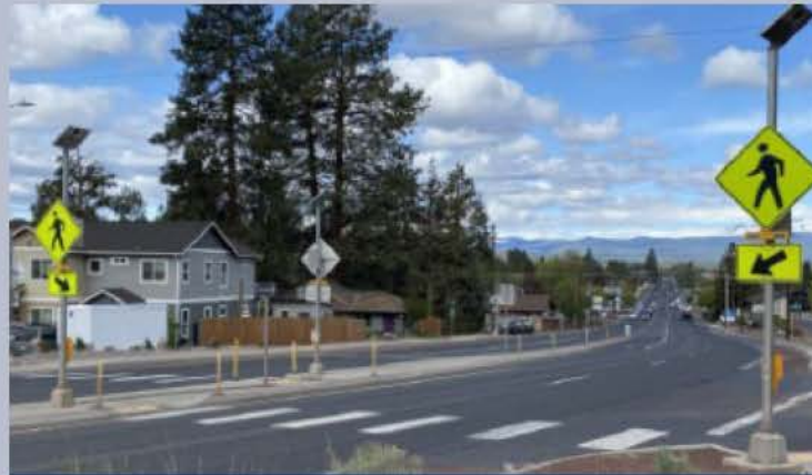
Rectangular Rapid Flashing Beacon (RRFB)
